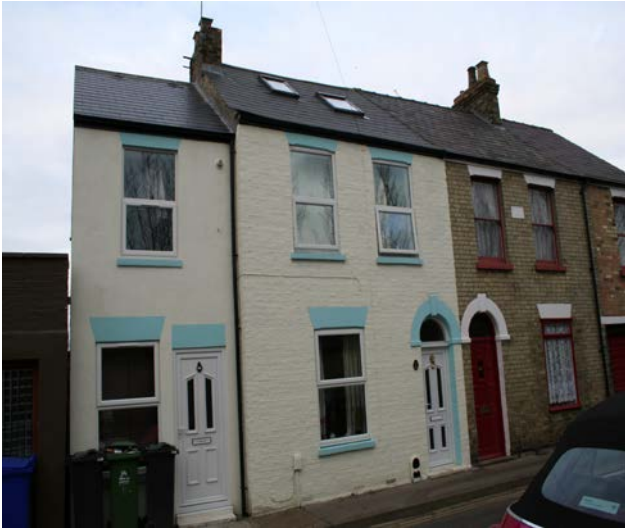
Poor replacement doors
